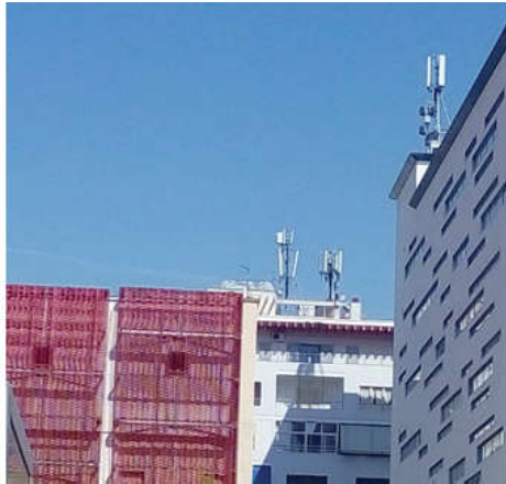
Figure 3- The cell phone antenna on the terrace of buildings (Vlore City)
