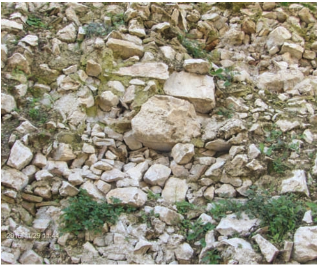
Photo.6 wall facade view with vegetation and potential collapsing stones
