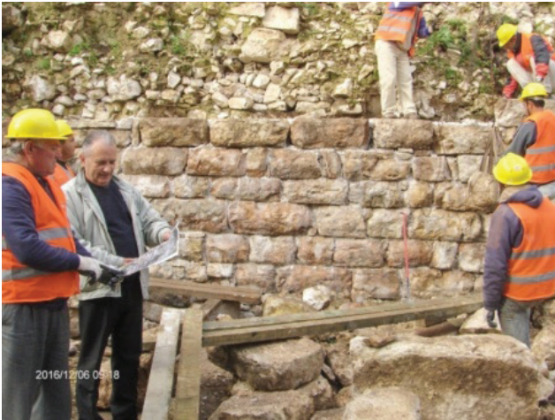
Consultation with the photo of the wall before the collapse, at the beginning of the restoration of each row.
