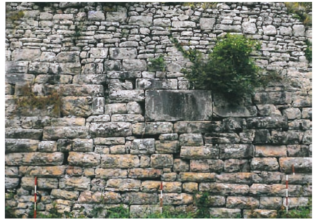
The facade of the wall before the collapse
