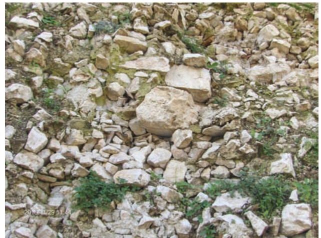
The facade of the wall after the collapse
