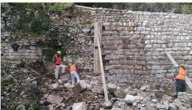
Photo 17-demolition of blocks risking to collapse and dissembling of the wall part near the southern wall
