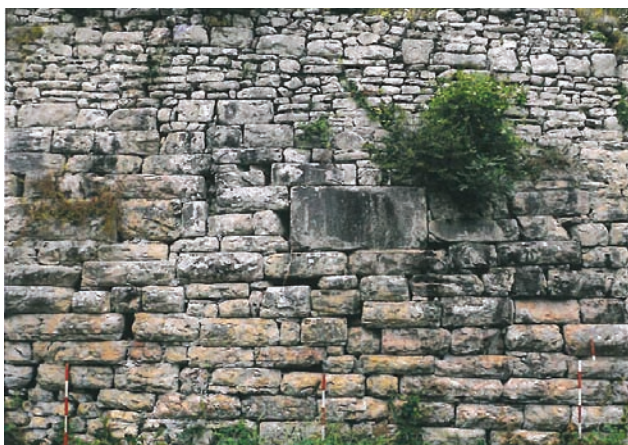
Photo 1-View of the wall before the collapse
